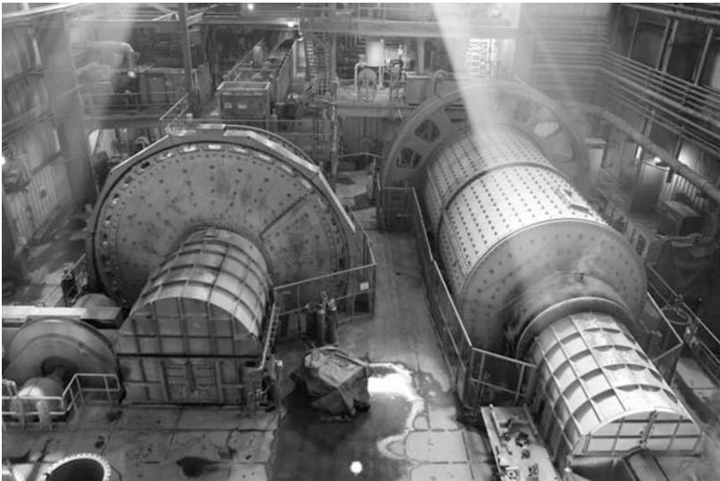
Grinding circuit in the Pogo Mill
