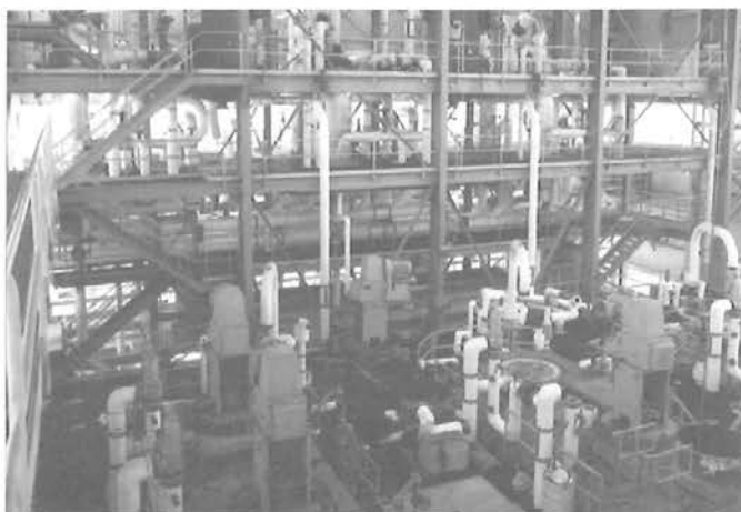
Autoclaves, slurry heaters, and flash tanks, McLaughlin Mine processing plant. (Courtesy of The Regional Oral History Office, The Bancroft Library, Berkeley, California.)
